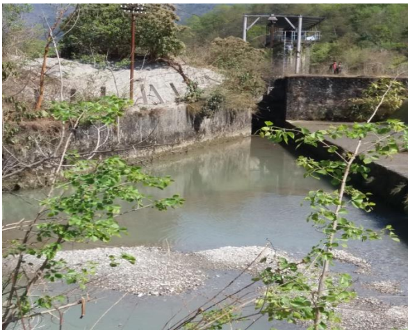
fig. Stoplog in forebay
