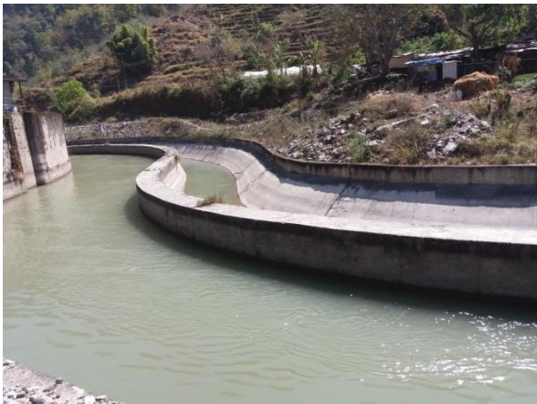
fig. Headrace canal and side canal
