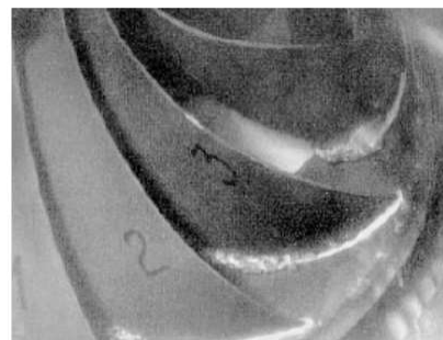
Inlet edge cavitation in Francis turbine
