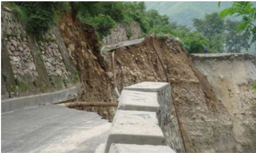
Damaged approach road, falling retaining wall and water supply line as on 27-06-2013
